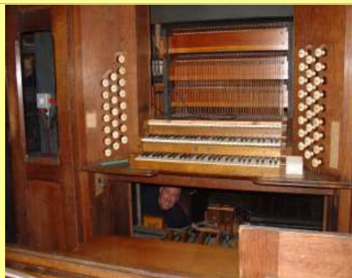
Plenty of work still to be done to prepare all the connections for the installation of the pedal board, currently being renovated. (Feb 2005)
